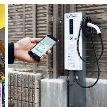
EV Stand (Installed at 313 halls)
