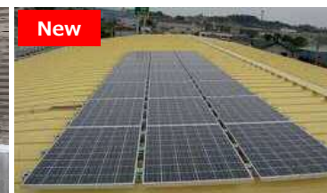
Solar Panels (To be installed at 40 halls in the 1st of this FY)
