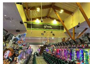
BEMS & LED Lights (Installed at all of halls)
